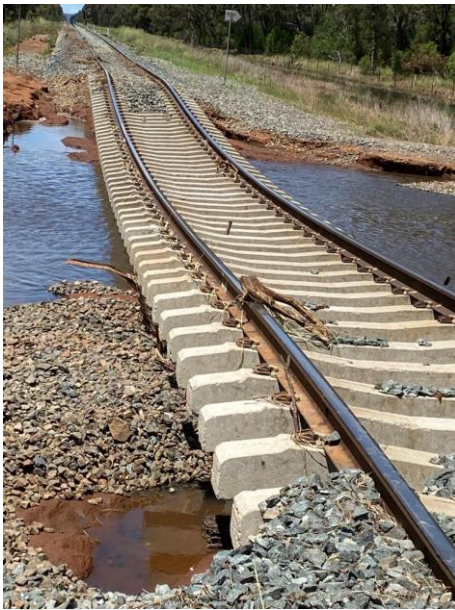
Plate C7.20 – Collapsed section of railway immediately to the east of Overland Road.
