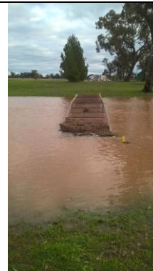
Plate C4.6 – Flooding in the vicinity of the 6 th fairway of the Bogan Gate Golf Club.
